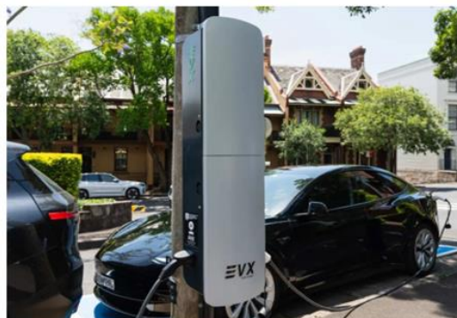
EVX's Pole mounted charging technology - Dual charging ports which allows for charging of two EVs from the same pole.
