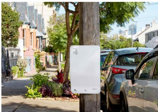
Intellihub's Power pole charger in NSW (ARENA Trial Project)
