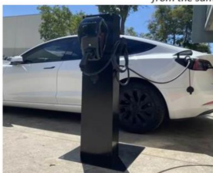
Kerbside (off pole) charger with both single and dual charge ports
