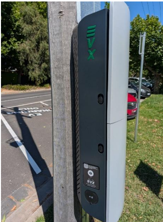
Pole mounted EV charger in Liardet St Port Melbourne
